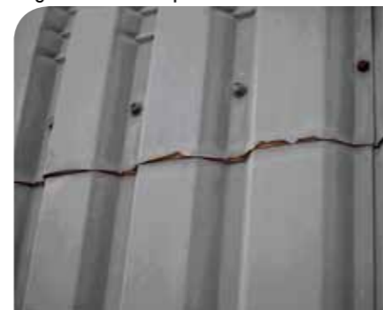
Typical example of cut edge corrosion
